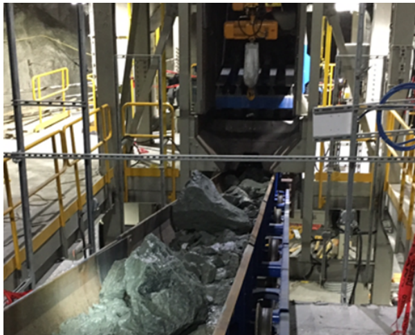
The Railveyor system is fed by a vibratory feeder system at Goldex. Other sites use more simple reclaim feeders, and many other feed options are available.
