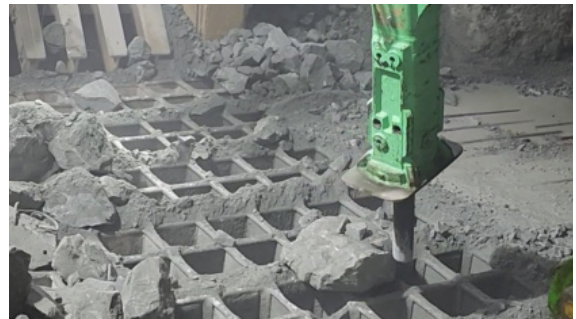
Rock breakers over a grizzly size ore which is then conveyed to the feeder that loads the Railveyor train.
